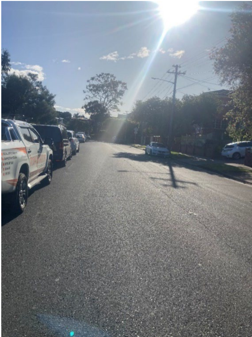
Figure 37 Faded Line Marking Henley Marine Drive
